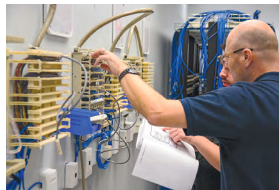
Hamilton, Ontario, Local 105 member Ashley Porter, left, and Thunder Bay, Ontario, Local 482 apprentice Louis Grenier go through network cabling specialist training at Local 402's training center.
